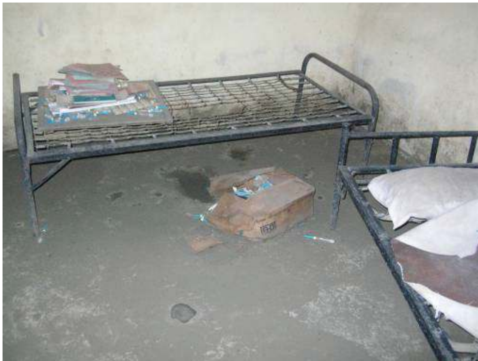
Overnight patient facilities in a comprehensive primary health care center run by Etche local government. The floors were caked with mud and strewn with vaccines ruined during a recent flood. The center had no mattresses, toilet facilities, or other basic amenities. © 2006 Chris Albin-Lackey/Human Rights Watch
