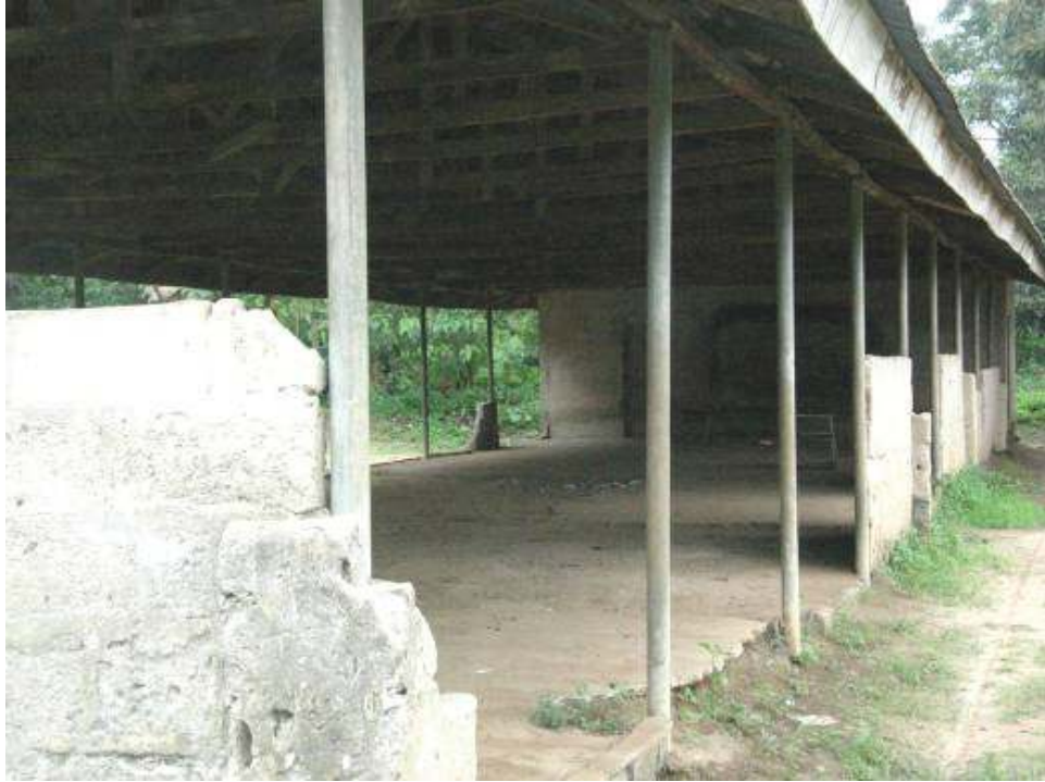
Block of primary school classrooms, Ulakwo, Etche local government. The school had no desks, no chairs, no teaching supplies and this classroom block had almost no walls. © 2006 Chris Albin-Lackey/Human Rights Watch
